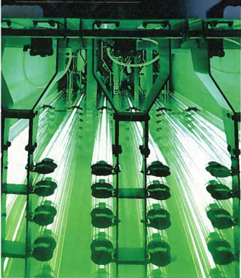
Gary Hengst checks a UV disinfection channel at the Lincoln facility.
